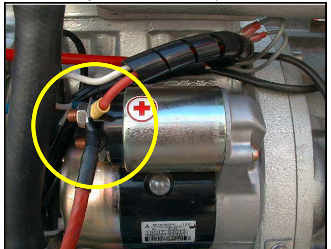
Fig. 7.12.1-1: Positive Battery Cable
