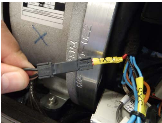
Fig. 13.5-1: Not Stop bridge in the cable harness
